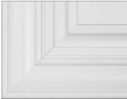
Example of door front joint separation
