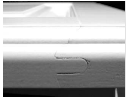
Example of door end joint separation
