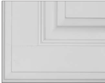
Example of door front joint separation
